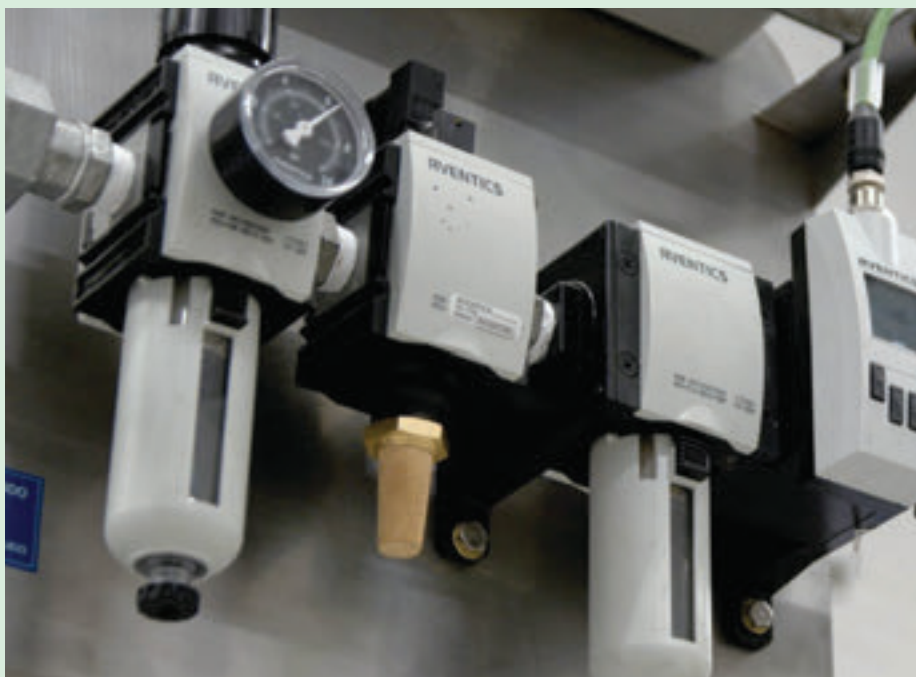
Colgate-Palmolive is using Emerson Aventics smart flow pneumatic sensors and IIoT-enabled software to monitor compressed air flow in real time.
