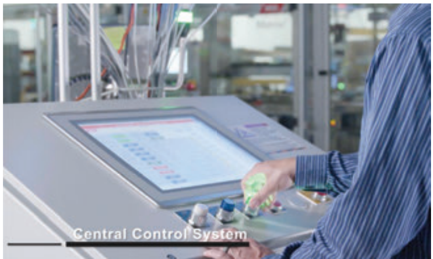
↑ The MGS Central Control System offers central control and monitoring for the entire line as well as final integration of the Optel Serialization System.
