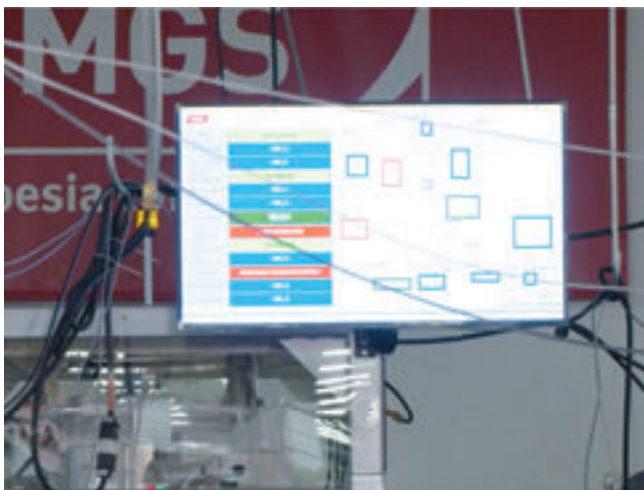
↑ Marquee Display Monitors allow operators to see real-time data for the entire system.
