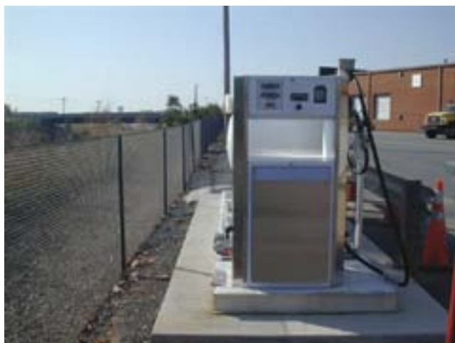
McCoy's Lawn Equipment Superstore has begun working with CleanFuel USA to upgrade existing propane refueling stations at both of its locations with liquid propane dispensers like this one.
