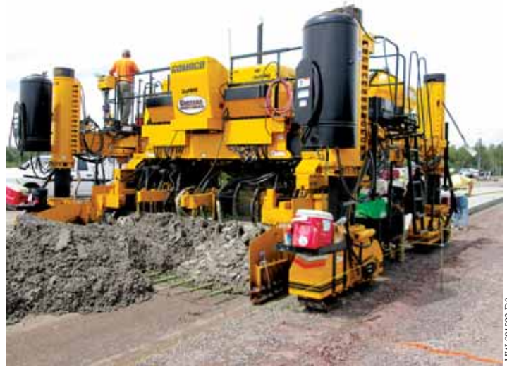
The Smart Width provides easy, accurate width change setup and also a reference for G+ to control proper steering and track speeds at varying widths of the paver.
