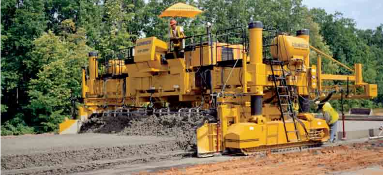
This two-track GHP-2800, equipped with an open-front mold, slipforms the concrete that was placed ahead of the paver over continuous steel on this mainline paving project near Lynchburg, Virginia.
