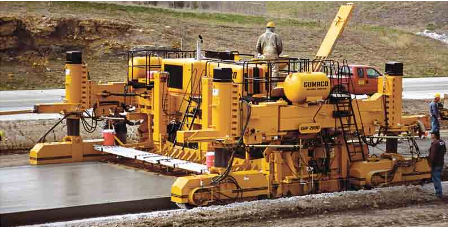
The GHP-2800 four-track machine provides high-production slipforming on this mainline highway project in Kansas City, Missouri. This highway was slipformed in passes 22 ft. (6.71 m) wide by 12 in. (305 mm) thick.
