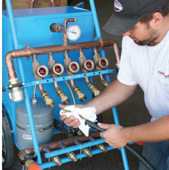
Clean disconnect prior to connecting to CCS.
