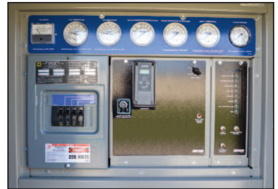
8-light diagnostic panel
