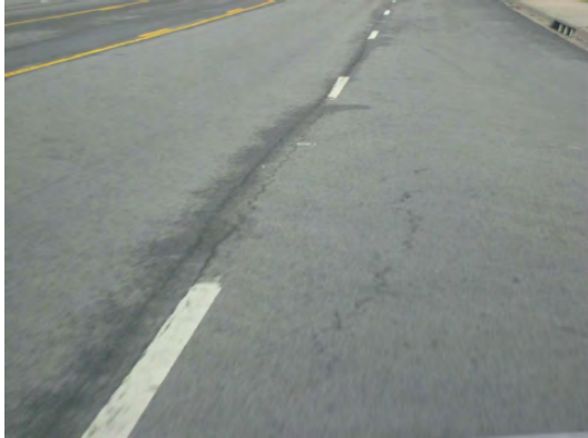
typical joint problem
